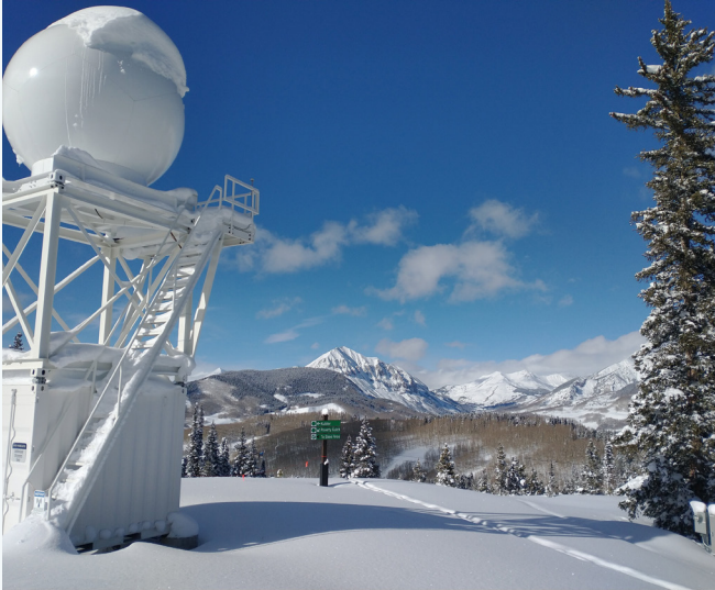
An X-band precipitation radar (XSAPR) is pictured on Crested Butte Mountain in Colorado as part of the SAIL (Surface Atmosphere Integrated Field Laboratory) campaign. Source: image courtesy of the DOE Atmospheric Radiation Measurement (ARM) user facility.
