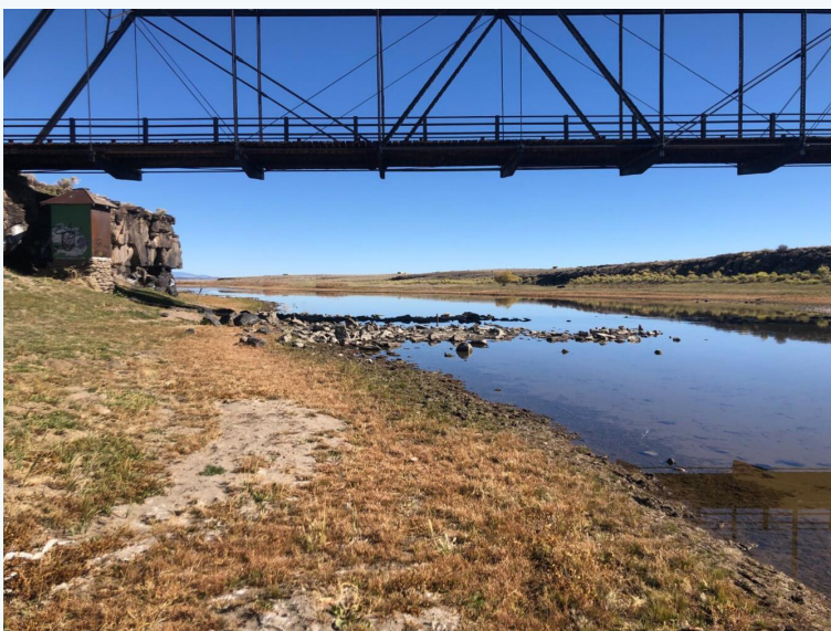
Upstream image of Lobatos stream gauge on the Rio Grande Source: USGS.
