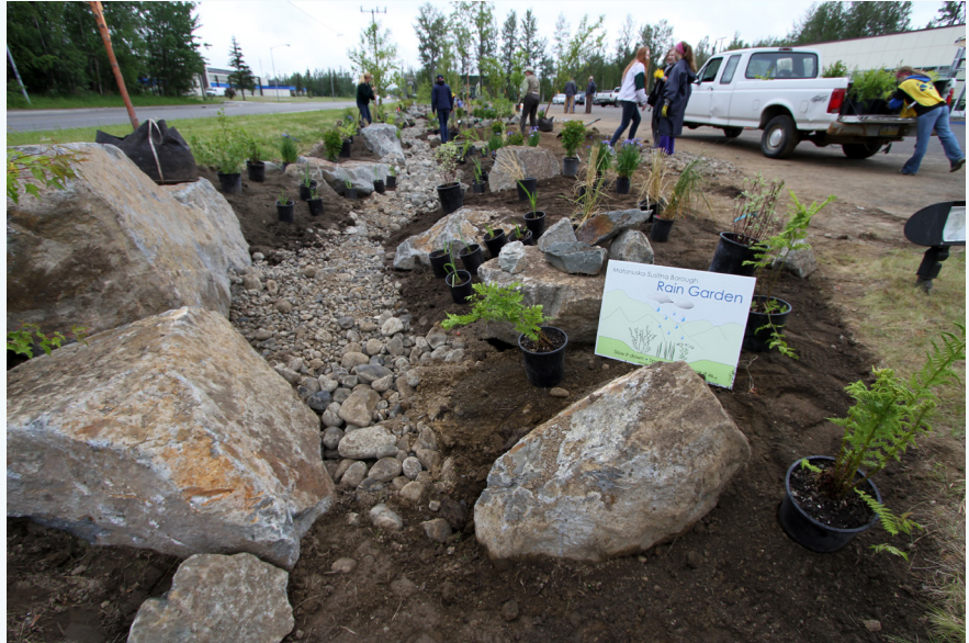
A rain garden being installed at the Palmer Senior Center in Southcentral Alaska to help manage stormwater runoff. Credit: USFWS/Katrina Mueller.
