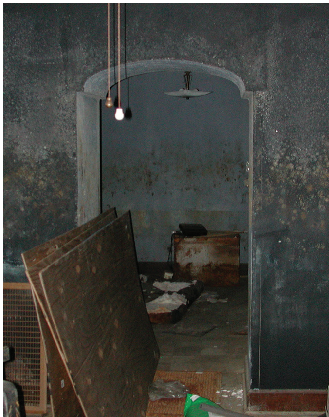
Dampness and mold in U.S. homes are linked to approximately 4.6 million cases of worsened asthma.
