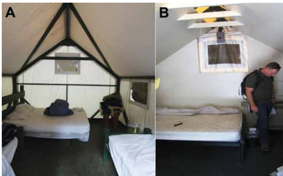
Figure 3. Inside view of regular and signature tent cabins, Yosemite National Park, summer 2012. A) Regular tent cabin showing canvas affixed over a wood frame. B) Signature tent cabin showing drywall between the exterior canvas and the interior living space.
